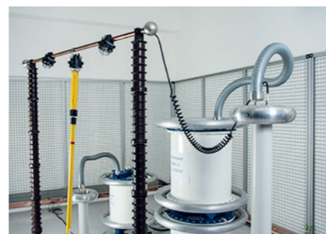
High voltage laboratory
